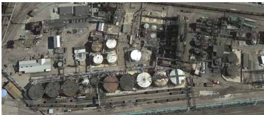
The former Koppers plant in Clairton, Pa., is currently undergoing a carefully phased demolition and dismantling process.
